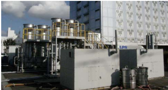
Groundwater decontamination equipment installed at the site (the Head Office)
