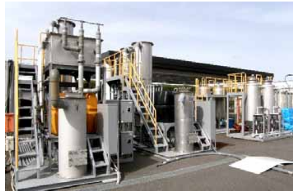
Soil decontamination equipment installed in the premises of the Head Office
